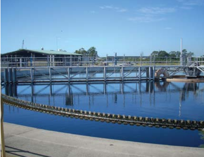
> Clarifier at Luggage Point Water Reclamation Plant, Queensland.
