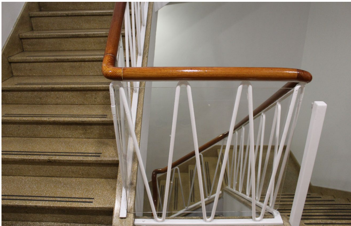
Figure 3.37 An original stairwell with terrazzo treads and risers. The balustrade has been brought up to code by installing a Perspex sheet.
