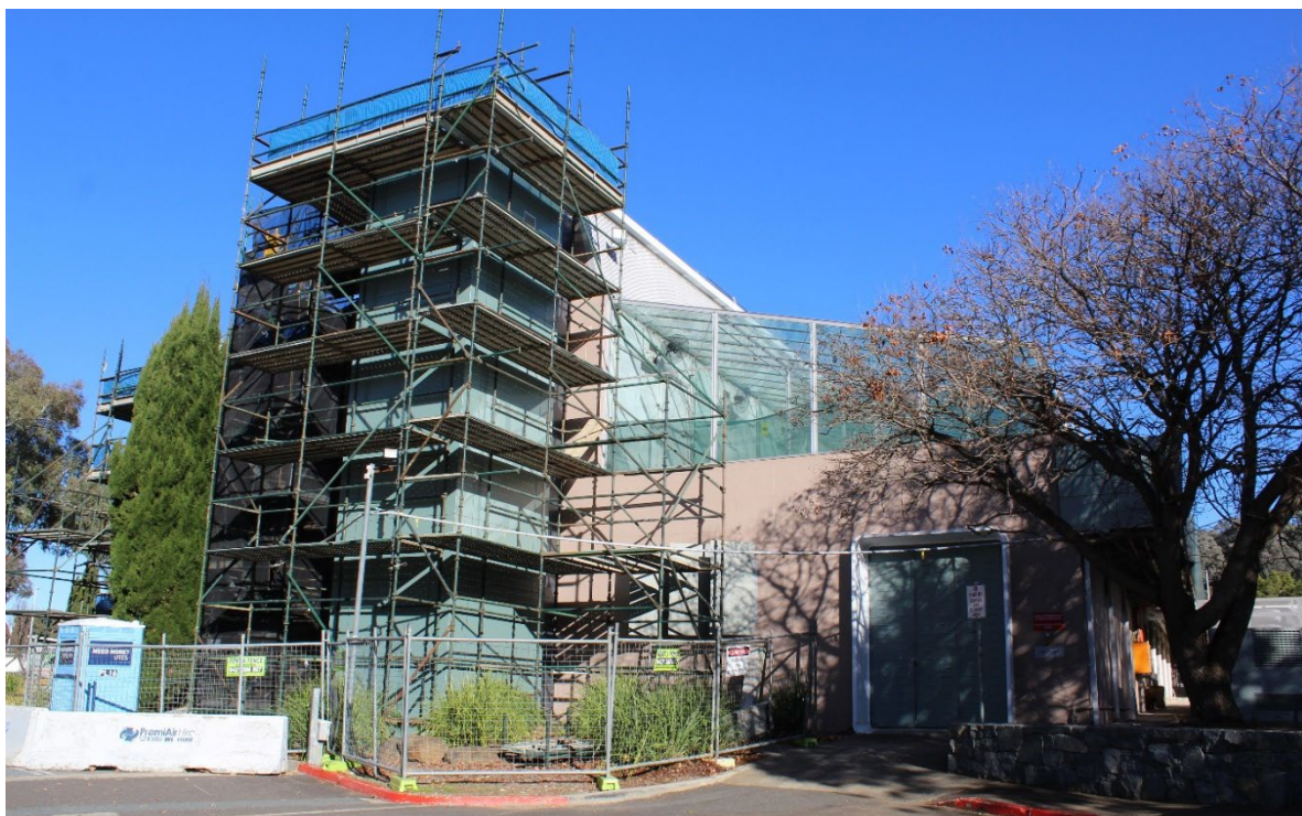
Figure 3.42 The eastern elevation of the Phytotron and Phenomics Centre. The lift shaft was installed in 2013. The scaffolding is associated with the 2023 roof sheeting replacement.
