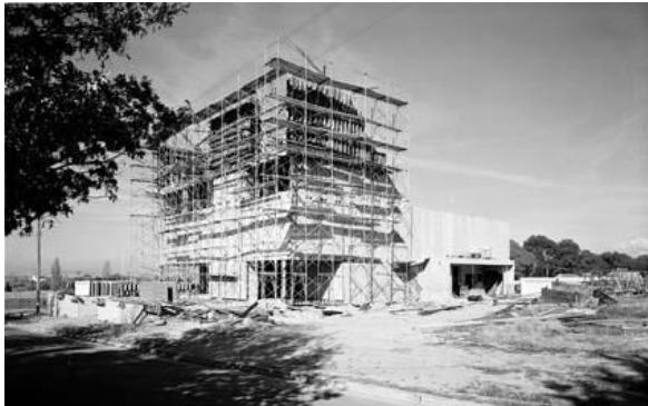
Figure 2.11 Construction of the Library (Building 060) in 1971. (Source: National Archives of Australia, Item ID 30108524)
