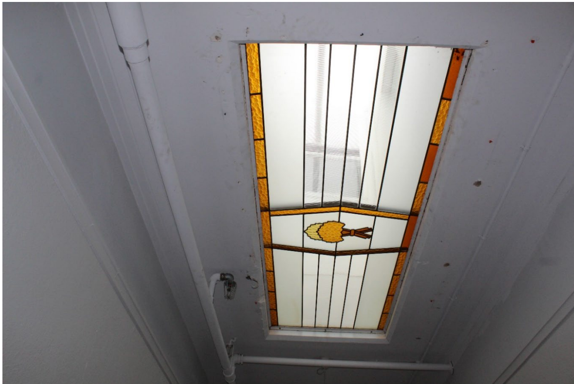
Figure 3.38 Coloured glass diffuser/skylight in the North Wing with the wheat sheaf symbol. The glass was fully replaced after the 2020 hailstorm.
