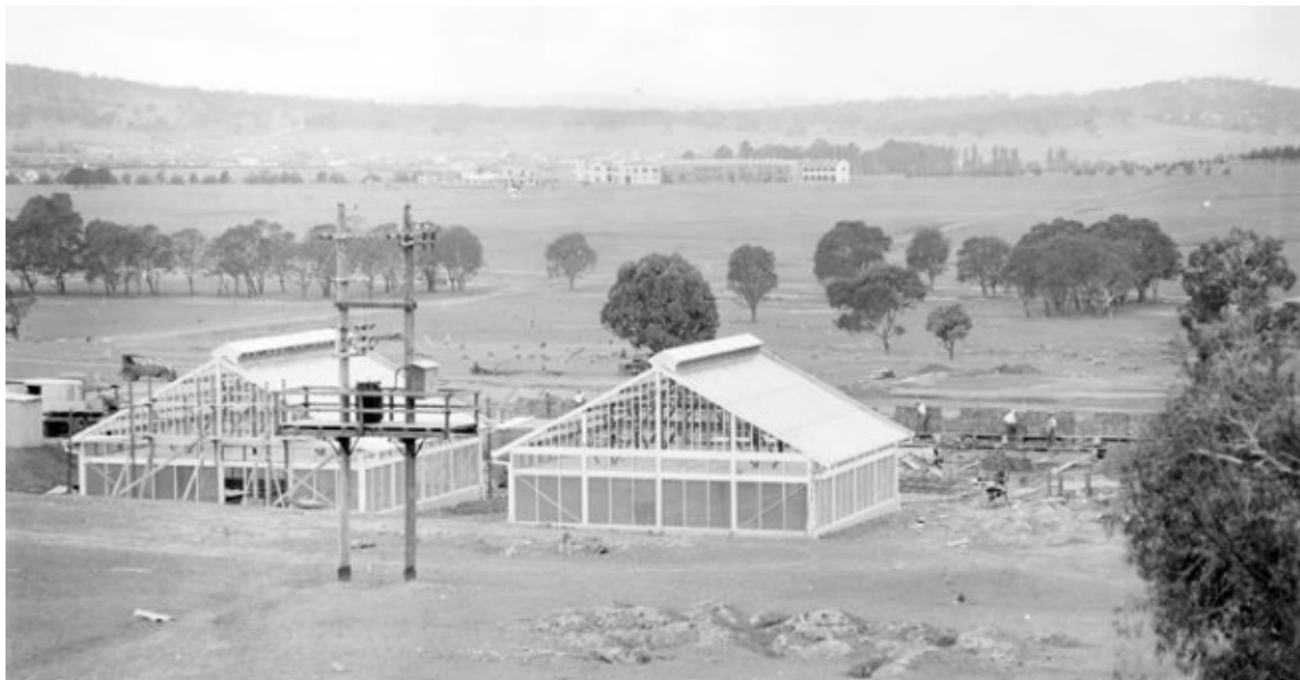
Figure 2.5 Two insectaries (Buildings 123 and 132, since demolished) during construction in April 1929. The Sydney and Melbourne Buildings on Northbourne Avenue are visible in the background. (Source: National Archives of Australia, Item ID 3151427)
