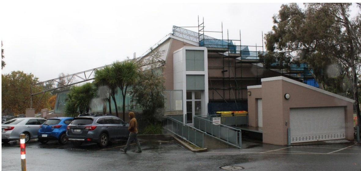
Figure 3.40 The western elevation of the Phytotron and Phenomics Centre. The cabbage trees ( Cordyline Australis ) are in the left of the photo.
