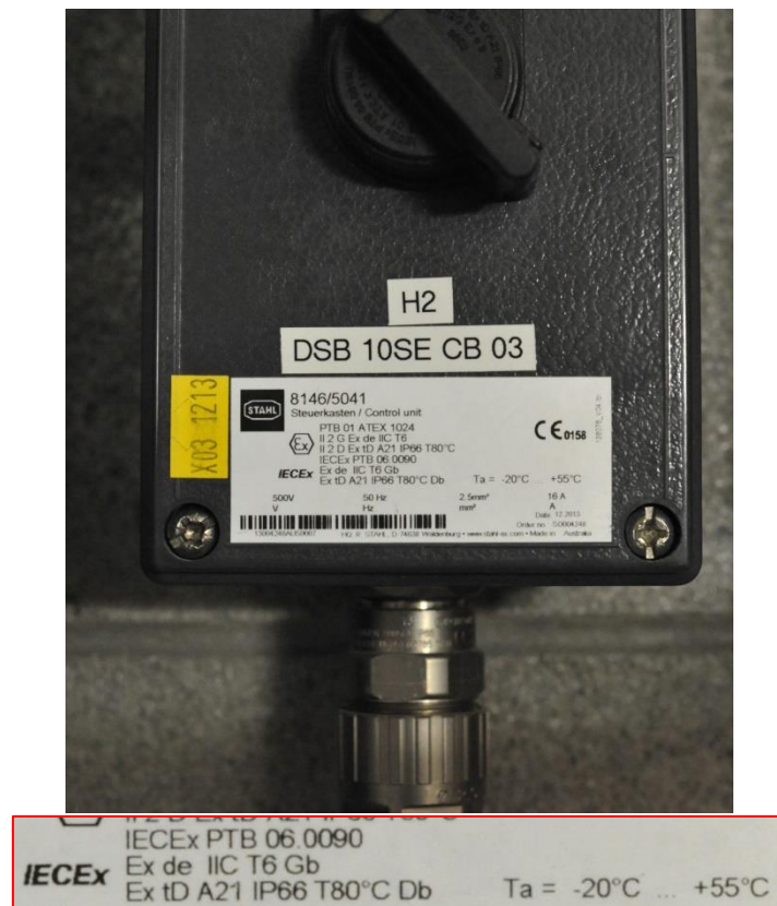
Figure 3 – Example of a Hazardous Area Rated Equipment Markings – Example 1 - Switch
