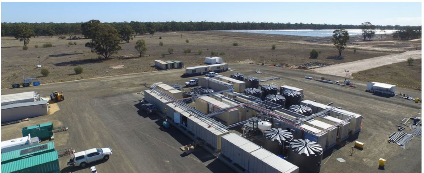
1.5 MLD Santos Leewood Desalination Plant near Narrabri, NSW with concentrate evaporation ponds in the background
