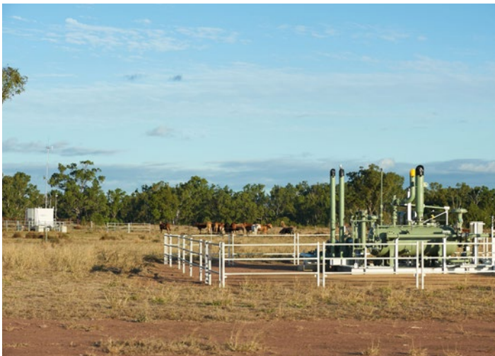
Coal seam gas well and an air monitoring station in the background.
