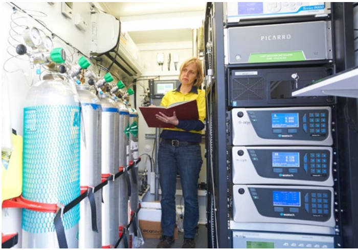
Air monitoring equipment inside the station.
