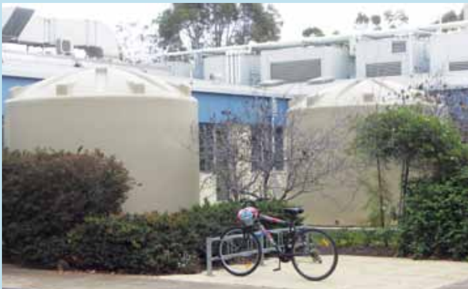
Some of the rainwater tanks located at CSIRO's Werribee – Sneydes Road site. Credit: Murray Brown
